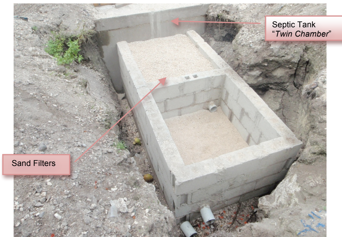
Figure 7 Prototype #1: A Conventional Septic Tank “Twin Chamber” added with two stages Sand Filters as Secondary Treatment to improve the waste water effluent prior being discharge via irrigation.
