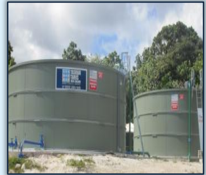
New 240kL water storage tanks
