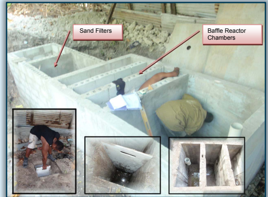
Improved septic tank with sand filter as secondary treatment prior to irrigation
