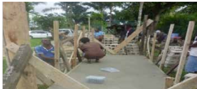
Above: Sanitation Enterprise Group building the compost toilet, laying the concrete base
