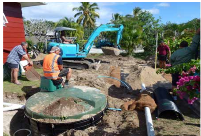
Above: Installation of package secondary treatment systems at a home in Muri, Rarotonga
