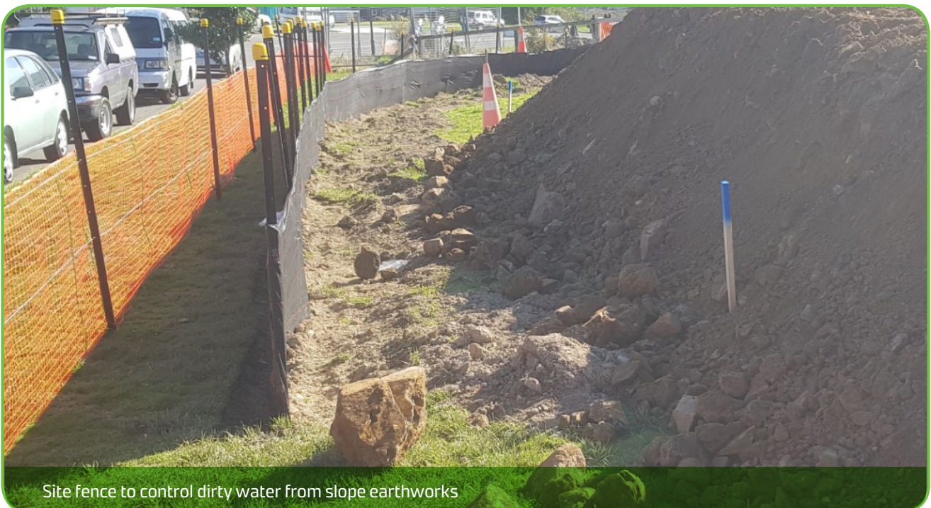
Earthworks (which increase site erodibility) carried out without sediment controls
