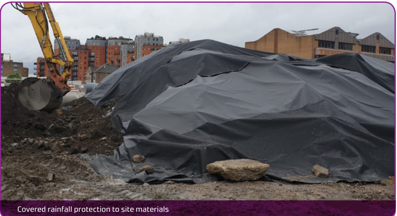
Stockpiled material for site without sediment controls
