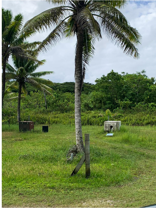
Figure 15: Water pump with transformer and black box Tusekolo, Alofi. Servicing Alofi north and Paliati area.
