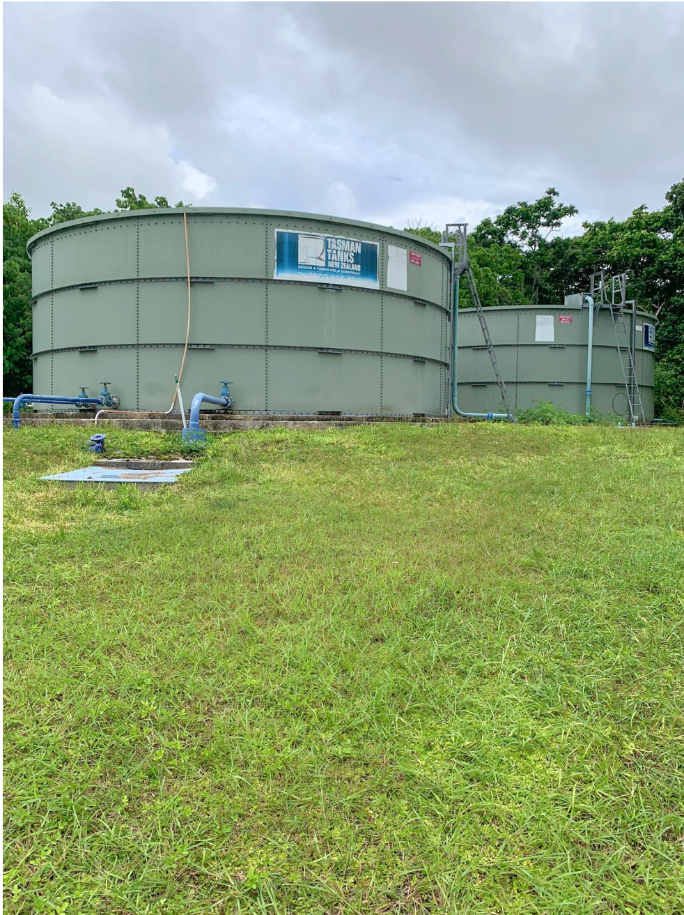
Figure 13: Twin new tanks at Tapeu servicing Alofi South.
