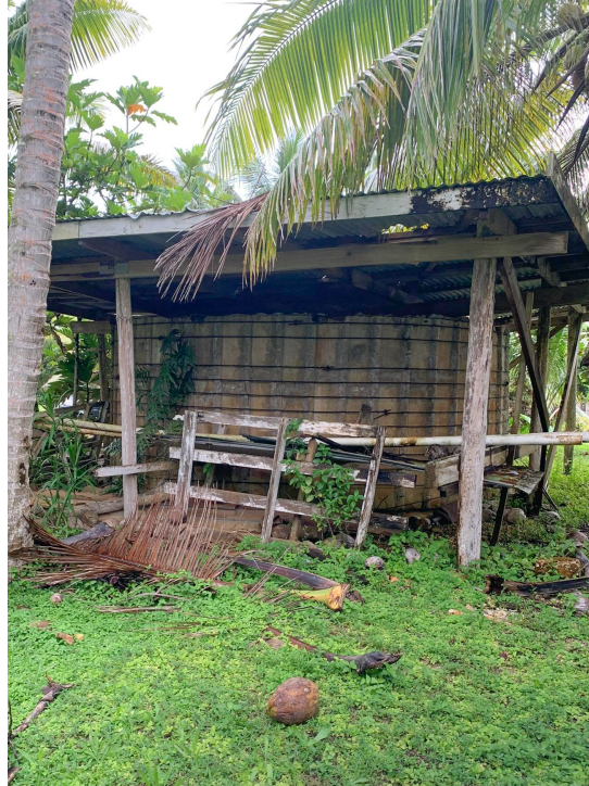
Figure 10: Concrete tank with old shelter at Liku (communal tank) before the windmills.
