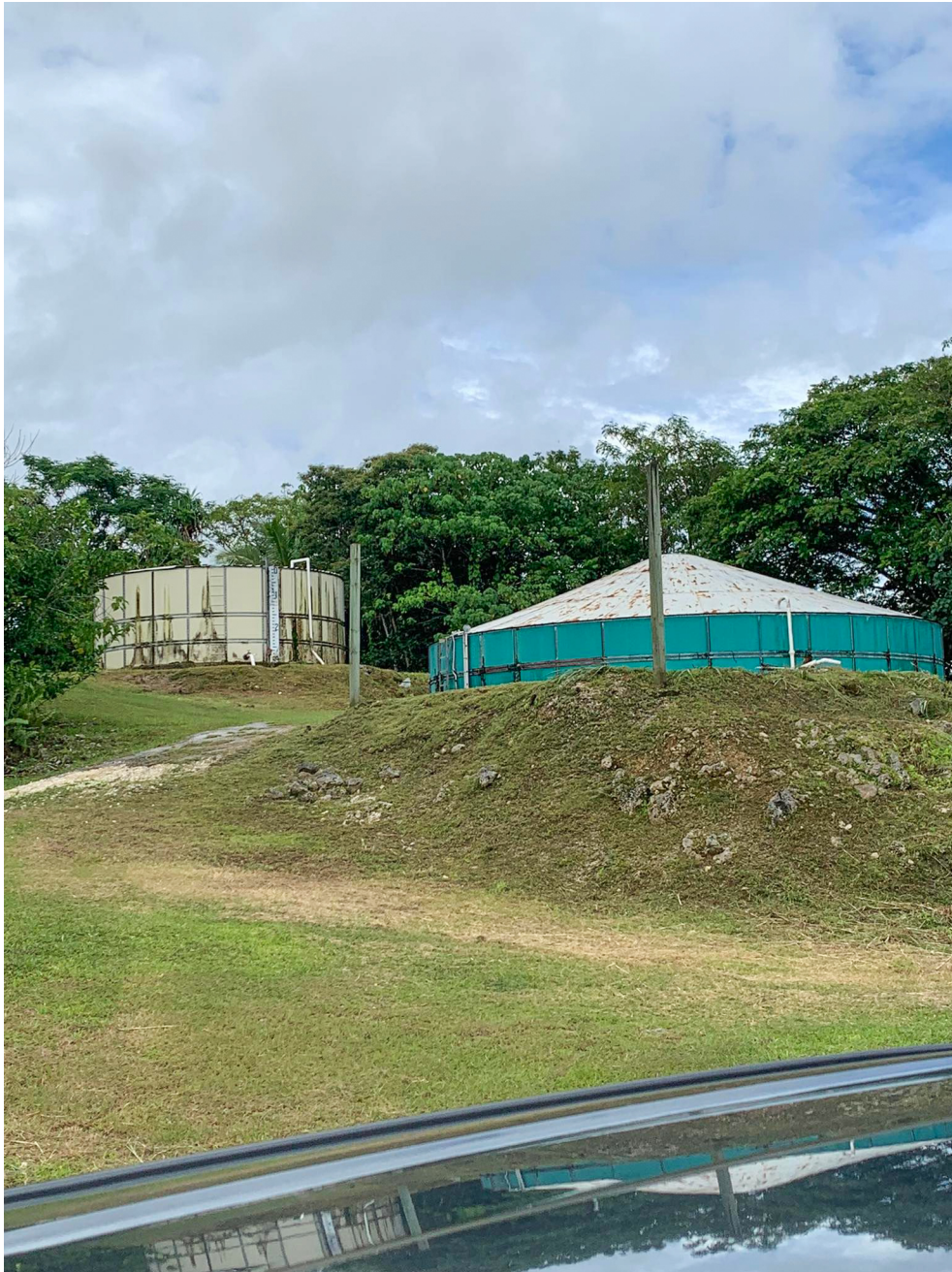
Figure 14: Twin green and yellow Paliati tanks servicing Alofi North.
