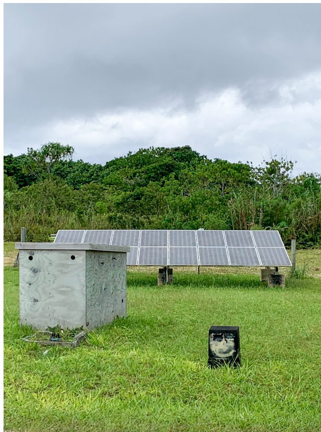
Figure 16: Water pump powered with solar panels at Fonuakula, Alofi.
