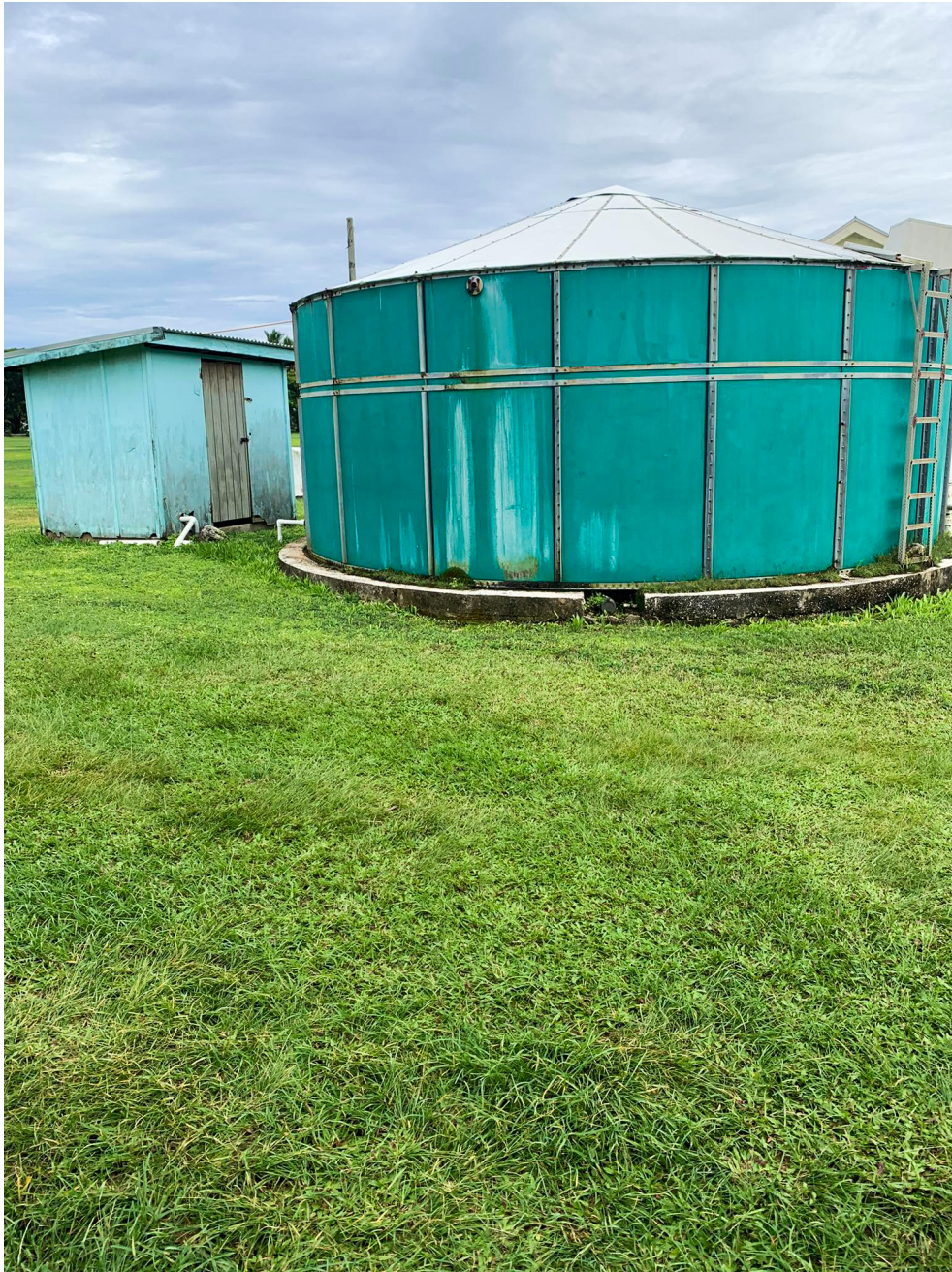
Figure 12: Green tank with pressure pump shed on the side in Liku.
