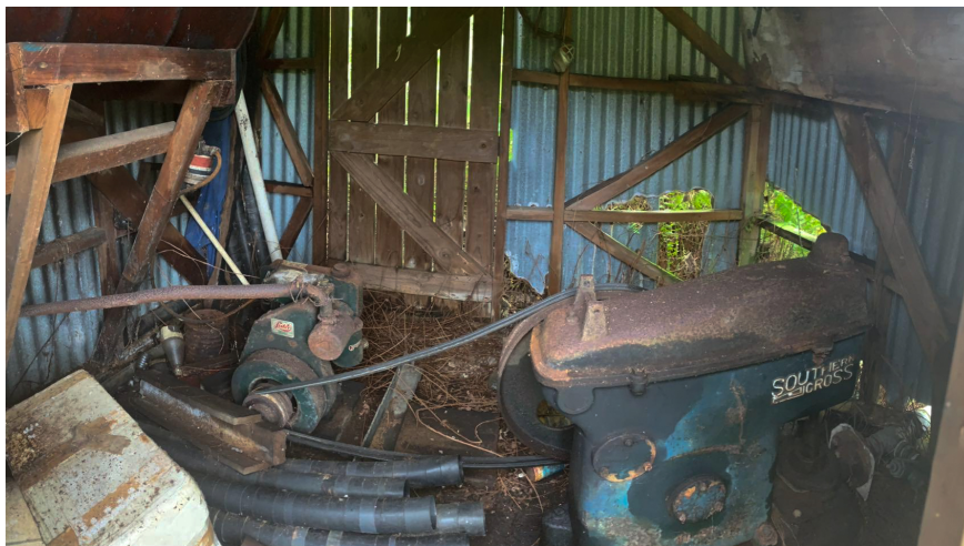
Figure 11: The Southern Cross diesel pump at Tumau, Alofi.
