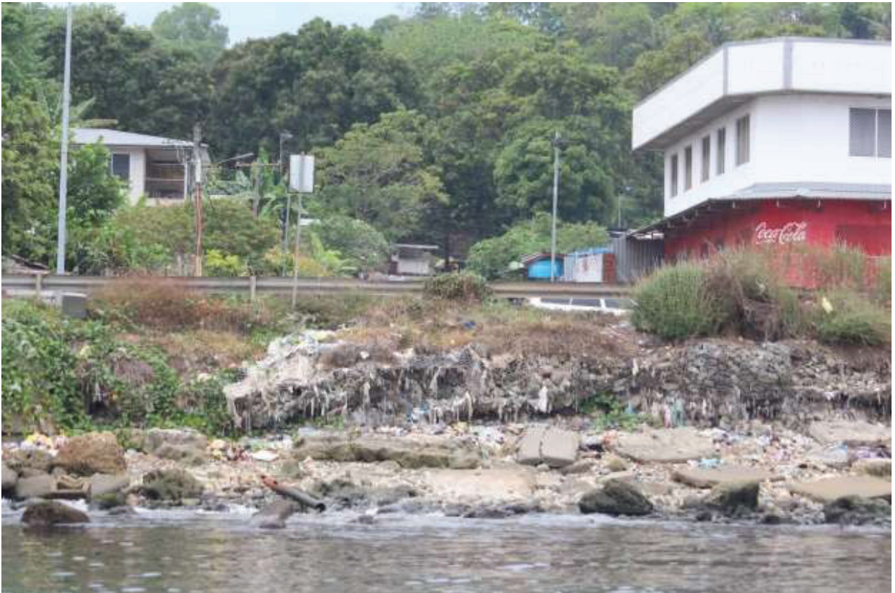
Image 1: Bahai road highway exposed to coastal inundation. Strong waves from cyclones and storm surges causes the built stone seawalls to rumbles away exposing the Main road connecting Honiara CBD and Ranadi. Image Courtesy: Danny Shadrech)
