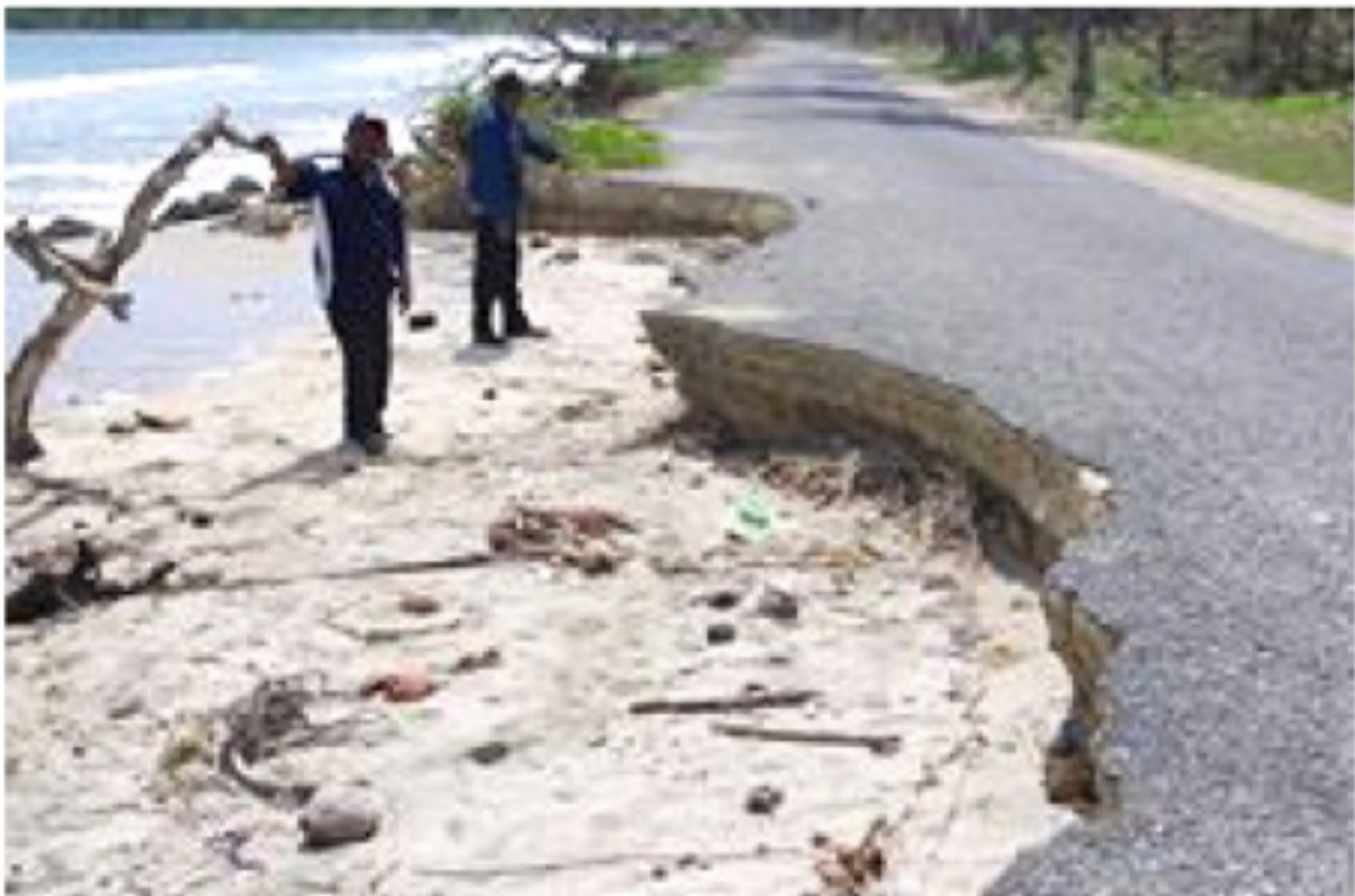
Figure 8. Coastal erosion at Wewak township
