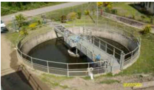
Sludge thickener at Matovo sewage treatment plant. Source: Matovo water safety plan.
