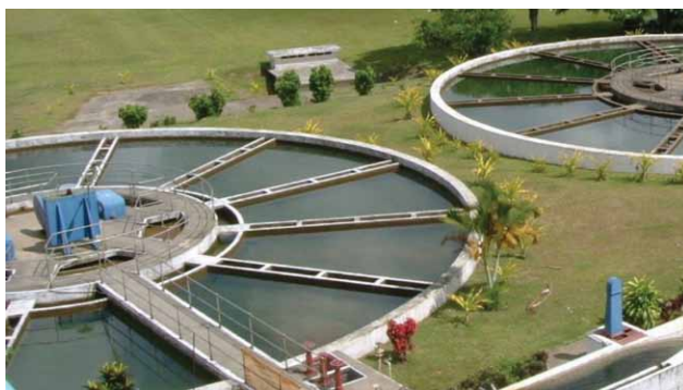
Treatment pools at Wailoku Water Treatment Plant. Source: Fiji Water Authority brochure.
