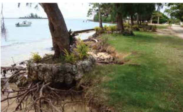
FIGURE 3-44 Erosion at lifuka
