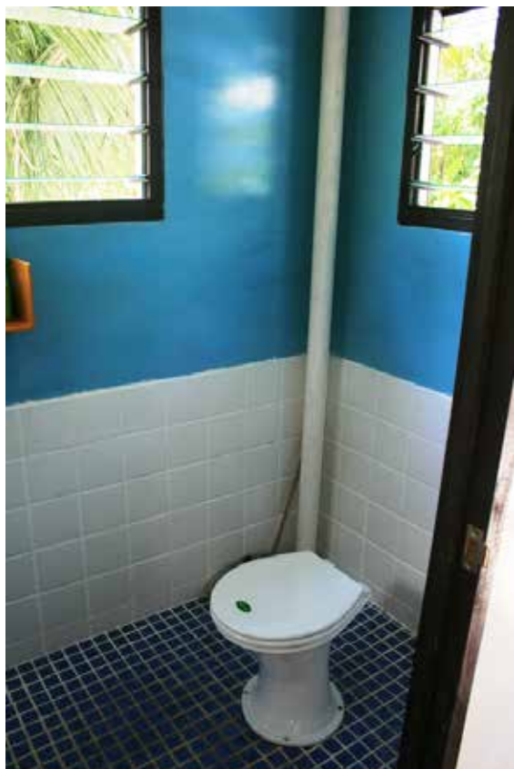
Figure 12: Waterless eco-sanitation toilet installed by the project
