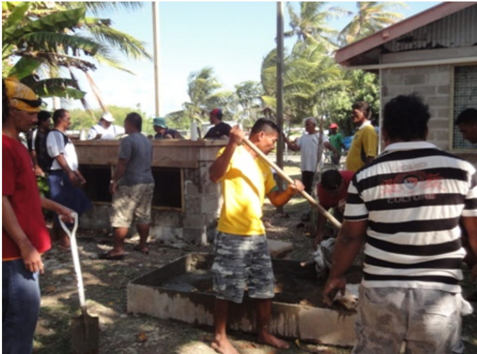
Figure 3: Construction workshop, convened for island construction workers to understand the principals of twin chambers and construct the toilets themselves
