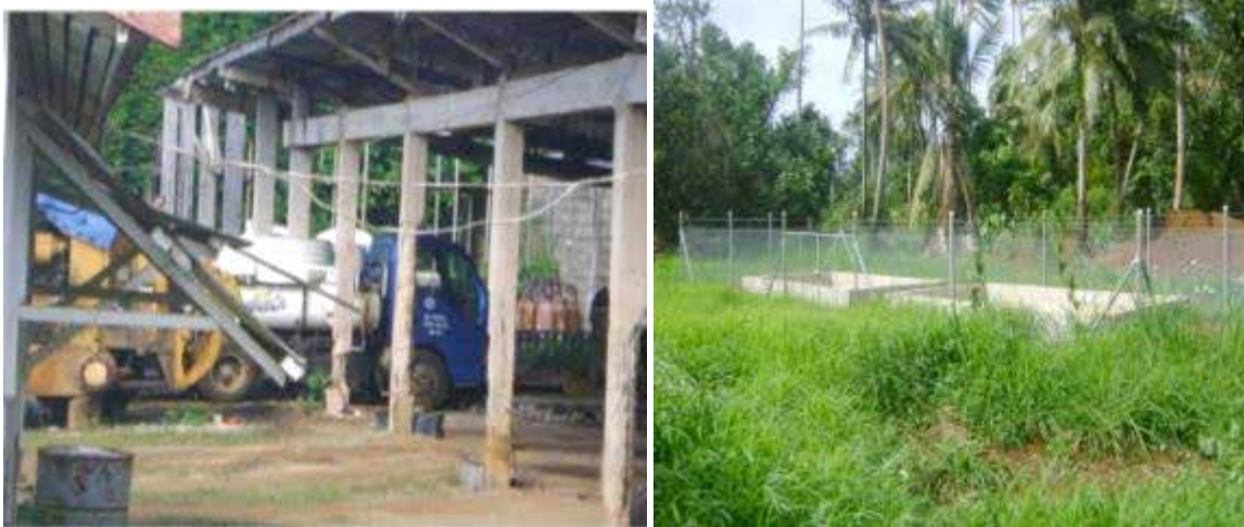
Figures 17 & 18: Vacuum truck and sludge management beds at Kalaka Site
