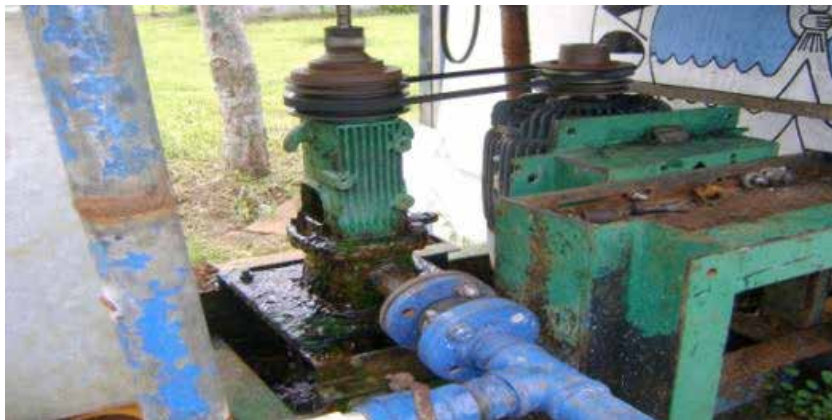
Figure 19 Old infrastructure associated with 70% leakage losses. A key study suggest that old valves may be contributing significantly to losses
