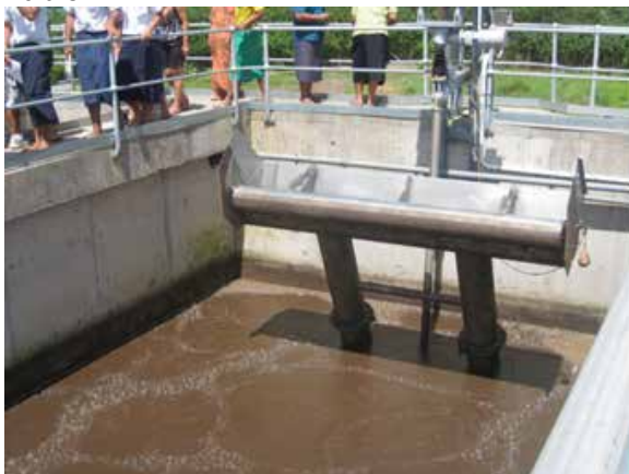
Figure 13 Waste Water Treatment Plant Sogi
