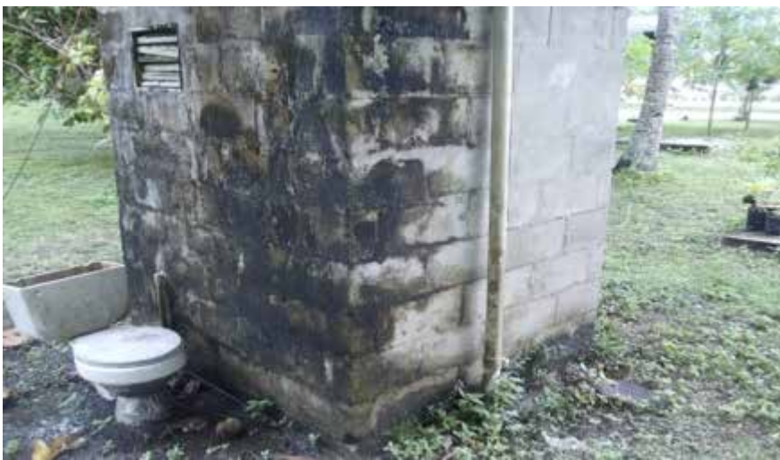
Figure 13 Current toilets being utilized at Laura providing poor sanitation and septic systems
