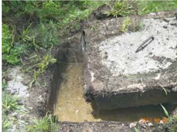
Figure 10: Example of an overloaded septic immediately above the Laura Water Lens
