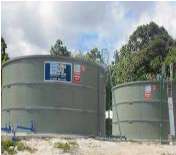
Figure 9: The two new 240 kL storage facilities at Alofi South
