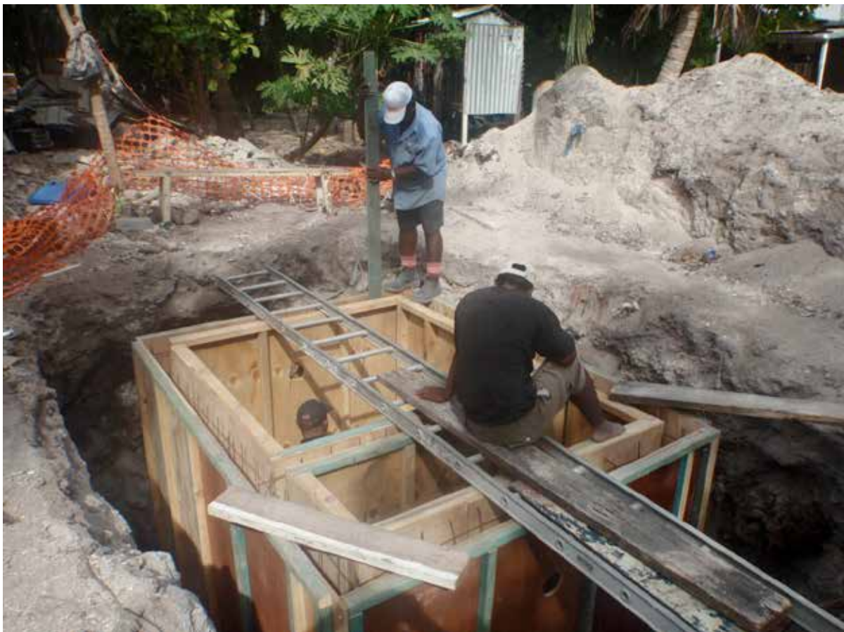
Figure 5 Contractor positioning the conventional Septic Tank mold at the demonstration community in Ewa. 22/02/2011.
