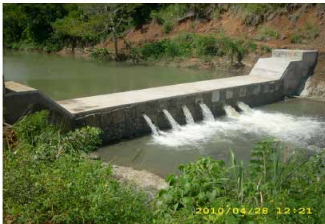
Figure 12: Retention Dam in the Upper Catchment – there are two more of the similar design
